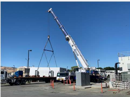
Delivery of New Electrical Switchgear
